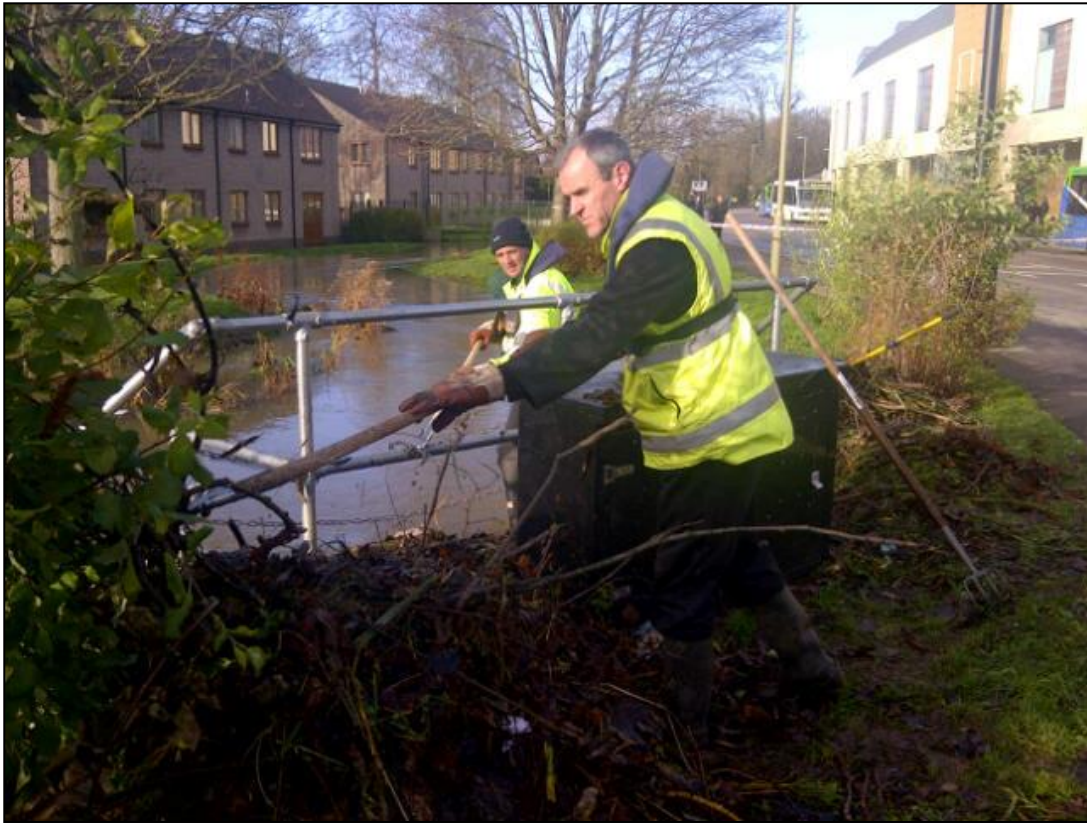
Figure 9: Environment Agency operational team removing debris from the River Bure trash screen at Hanover Gardens
